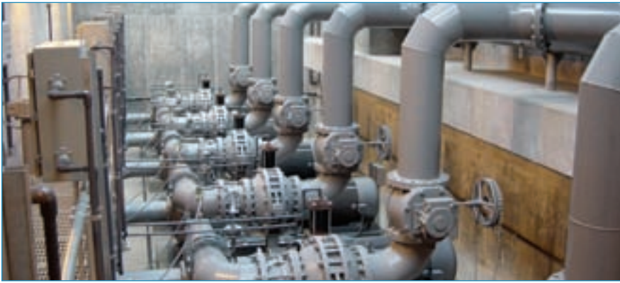
Pumps in the 36-mgd lift station that is the primary feed to the WWTP.
