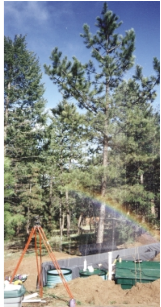
▲ During pressure testing, chambers disperse the effluent, transforming the high-pressure jets into a fine mist that will ensure unsaturated flow through the naturally sand media.
