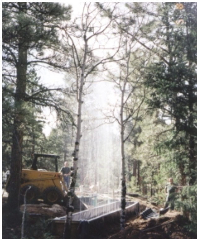
▲ Pressure tests were conducted on the polishing filter distribution network prior to placement of chambers.
