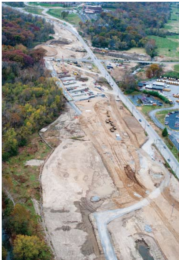
The Route 141 relocation project emphasized erosion control during the design and early construction stages.
