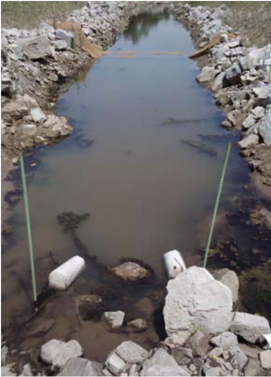
MoDOT used flocculant bags to remove extra sediment from water storage basins.
