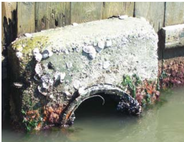
A storm water outfall in Ocean City, Md.
