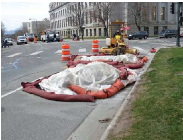
The location and scope of this high-profile sediment control project in Denver created many unique challenges, such as space concerns.
