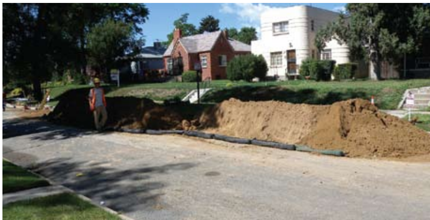
Due to the extent of impervious project area, vegetative buffer generally was not available.
