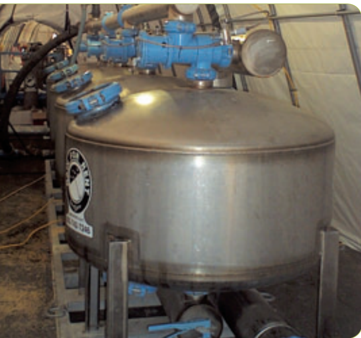
An active treatment sand filter system using a polymer
