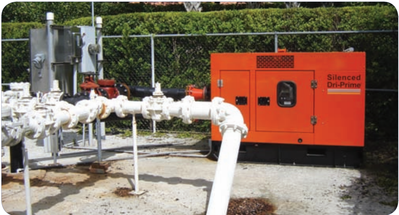
Backup pumping systems and lift station pump systems do not rely on one another to operate.
