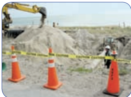
Two systems divert contaminated runoff into sand dunes.
