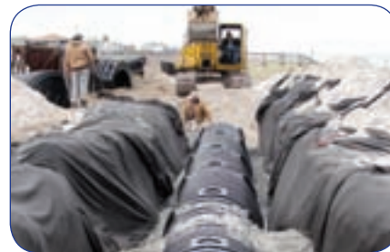
Kure Beach's storage and infiltration system promotes groundwater recharge.
