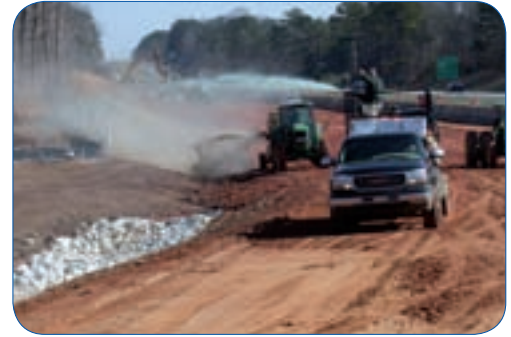
Pronto Grassing applies seed hydraulically before conducting a mulching operation on a busy Lee County project.
