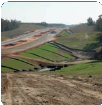
A Newell Roadbuilders Inc. project in Russell County makes good use of vegetation, earth berms, slope drains, silt fence and aggregate erosion control on the subgrade.
