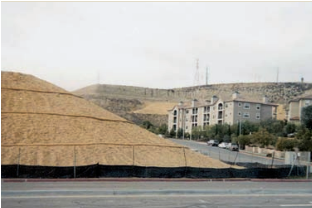
What little erosion this protected slope produces is effectively contained by the silt fence.
