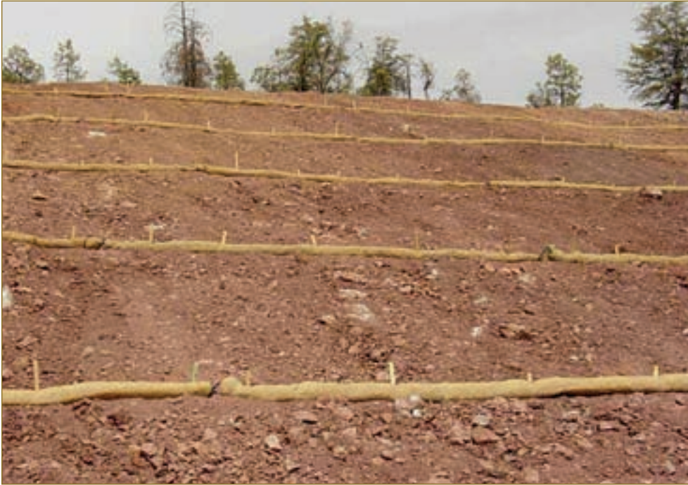
Fiber rolls placed along the contours of a slope face provide effective erosion control.
