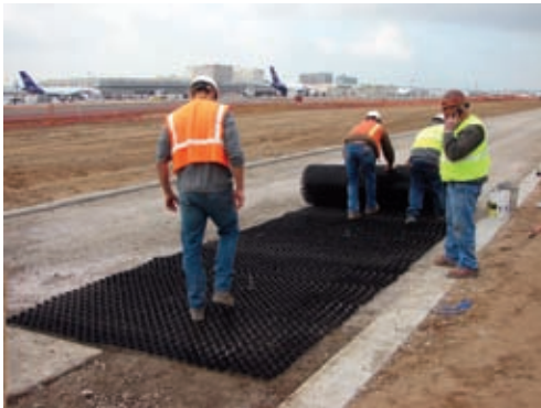
Construction crew members roll out porous paving system units at LAX and top them off with clean sand.
