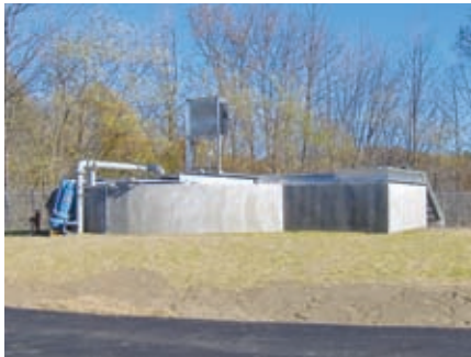
A view of Saco's new CSO treatment system.
