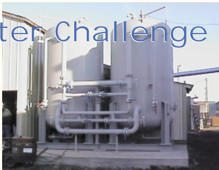
This system arsenic- and copper-removal system surpassed the required performance goals reducing both copper and arsenic to non-detectable levels.
