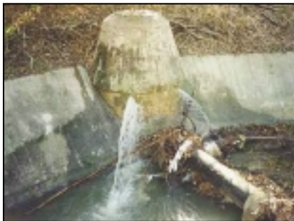
▲ This manhole, discharging sewage into the adjacent stream, depicts the environmental concerns associated with poorly managed sanitary sewer systems. By discharging raw sewage into the environment, sanitary sewer overflows pose a direct threat to human health.
