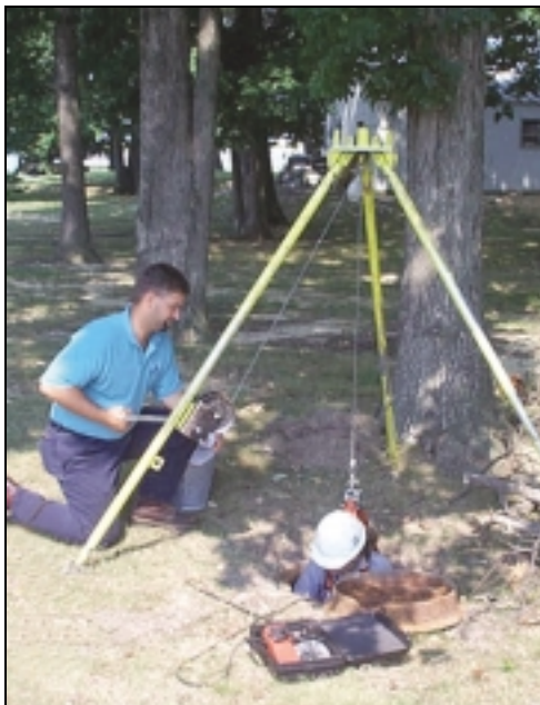
► Manhole inspections provide a general assessment of the sanitary sewer system manholes and identify active and inactive sources of inflow and infiltration.
